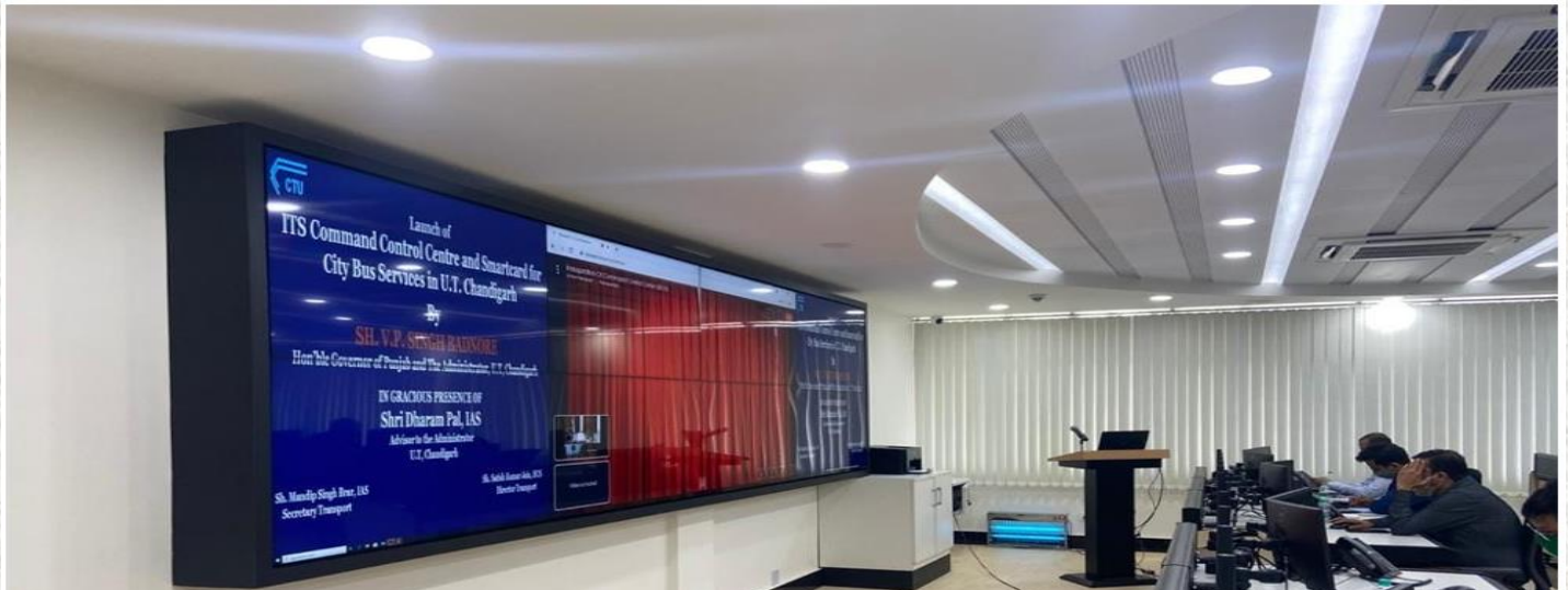
Real Time Monitoring & Tracking of Fleet at Command & Control Centre (CCC), Chandigarh Transport (CTU) with Chemito Intelligent Transport System (ITS)
